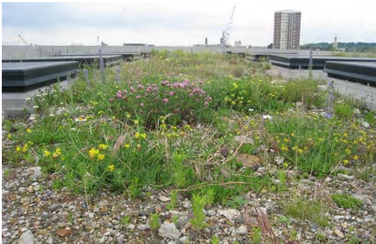
Figure 4-6: Example of naturally colonising brown roof on similar substrates to the Project Site
